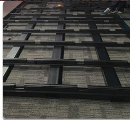
Fixed guide rail
